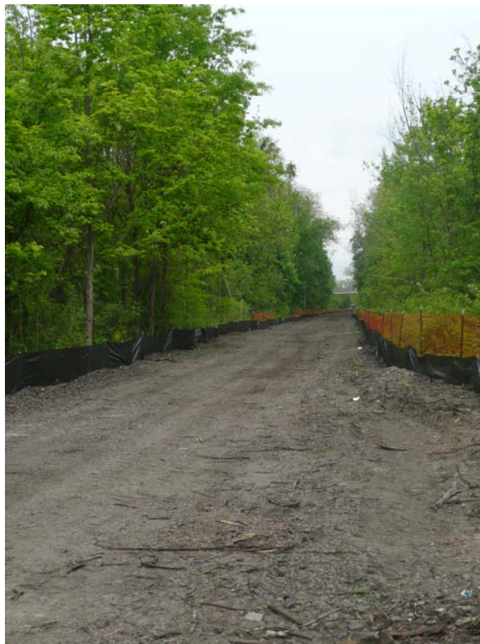
View of the Dutchess Rail Trail looking north from Overocker Road in the Town of Poughkeepsie. Paving on the main section of the trail will begin over the next few weeks.
